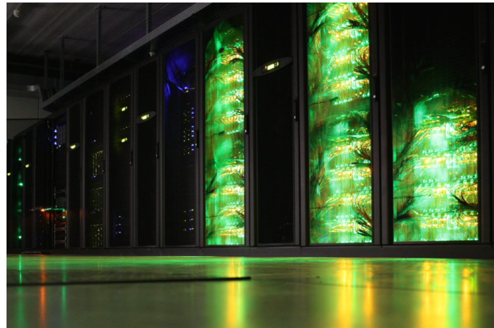
HPC-UGent Tier-2 infrastructure (ca. 2018)
