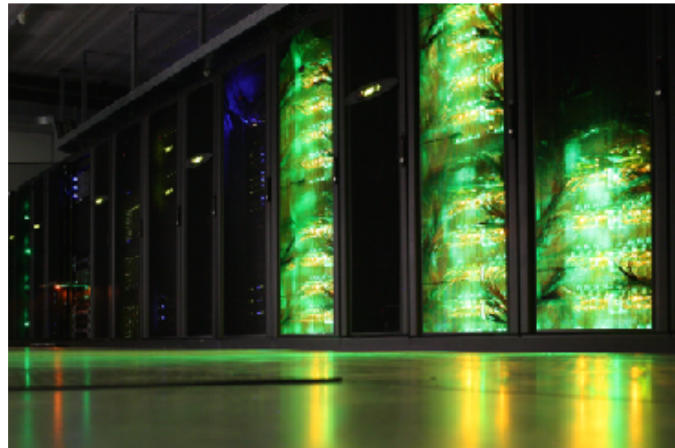
HPC-UGent Tier-2 infrastructure
